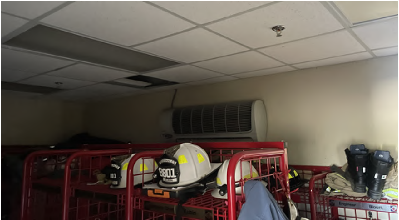
Figure 12 – Storage Room Mini-Split
