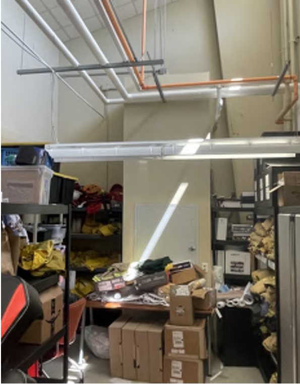
Figure 20 – Mezzanine showing dumbwaiter that requires removal.
