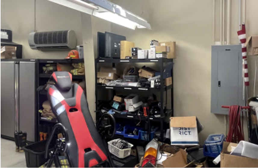
Figure 18 – Mezzanine with Mini-Split and Panel LE
