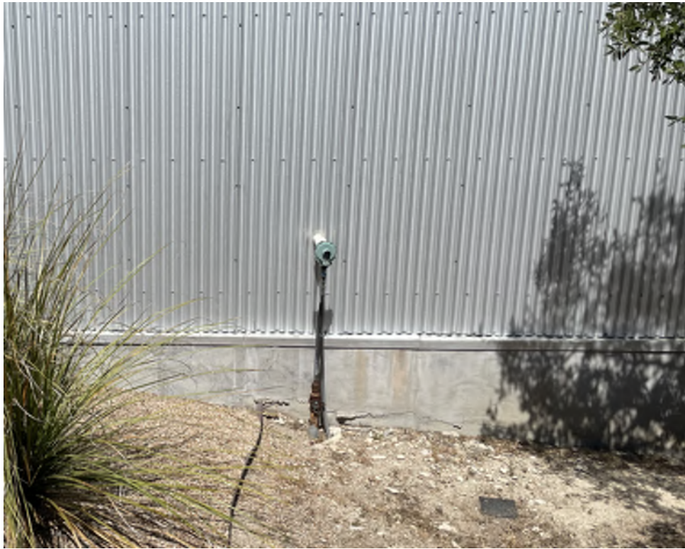
Figure 5 – Propane regulator and line up from buried propane tank.
