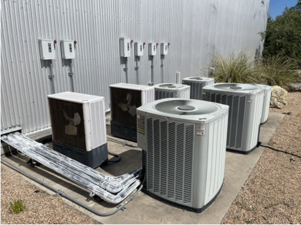
Figure 4 – Existing Condensing Units and Pad
